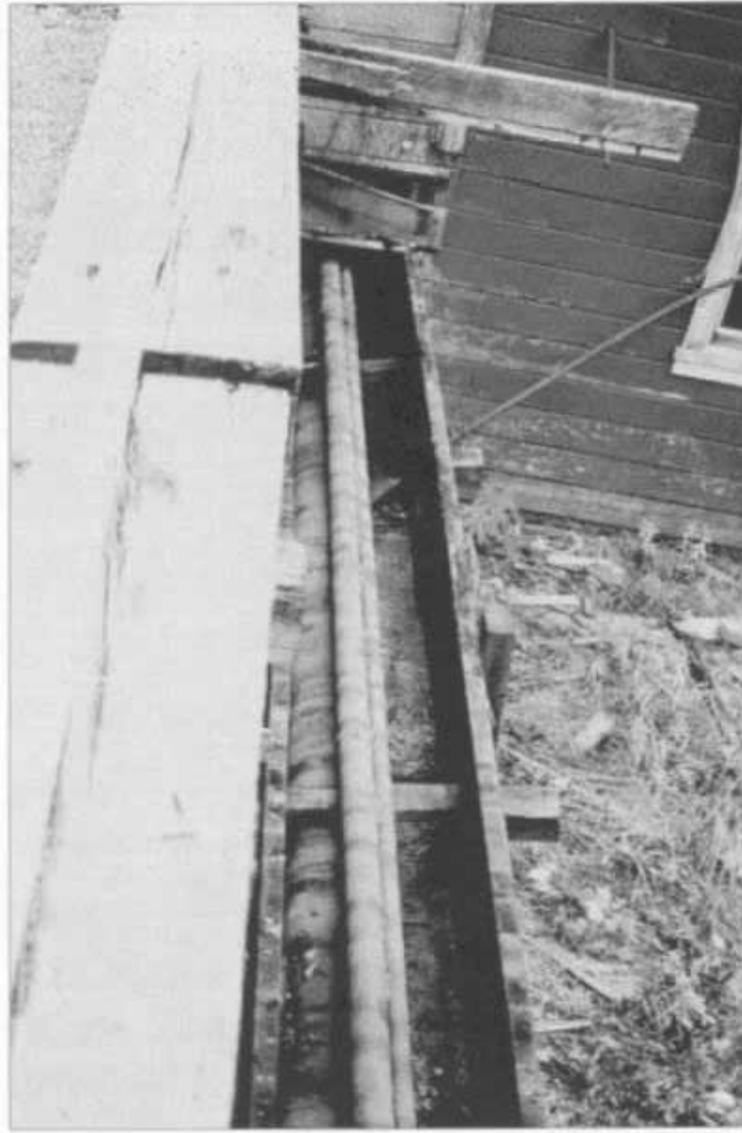
Many of Kennecott's utilidors were once insulated with asbestos
