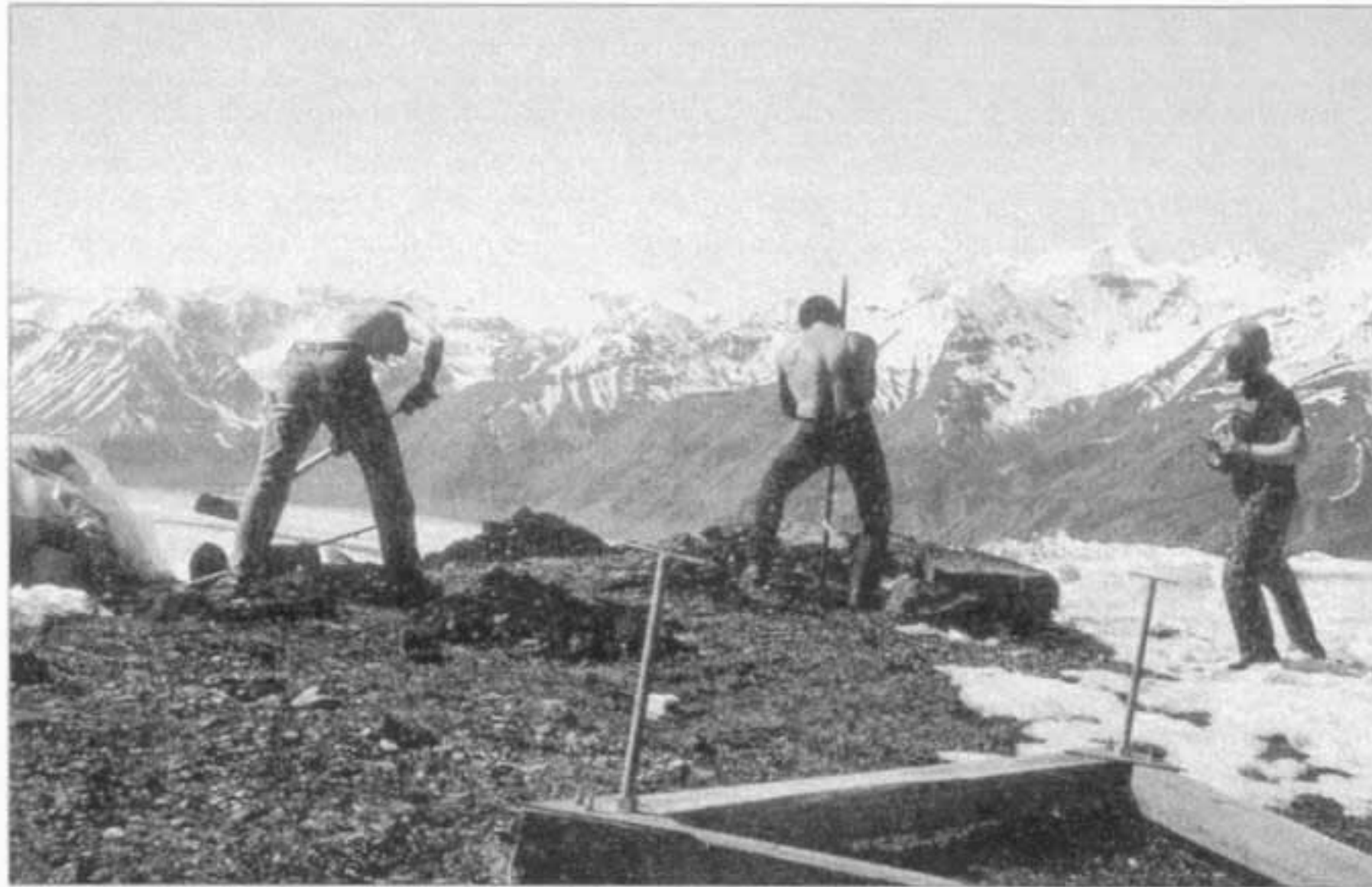
WRST crews prepared the repeater sites, like this one on Euchre Mountain
